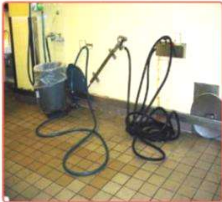
Uncoiled hose in a walkway
