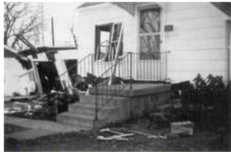
Low-Order Damage in a Dwelling.
