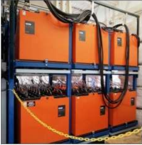
Typical Battery Installation for a Photovoltaic Solar Power System
