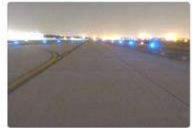
Blue taxiway edge lights
